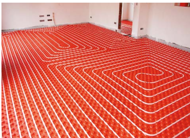
Photograph 2.2: Built-in electric system
